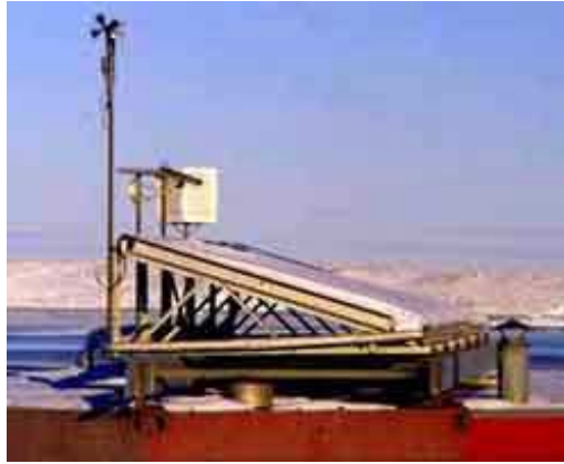
Figure 4.8: The solar thermal system installed at Australia's Davis station (AAD, 2005)
