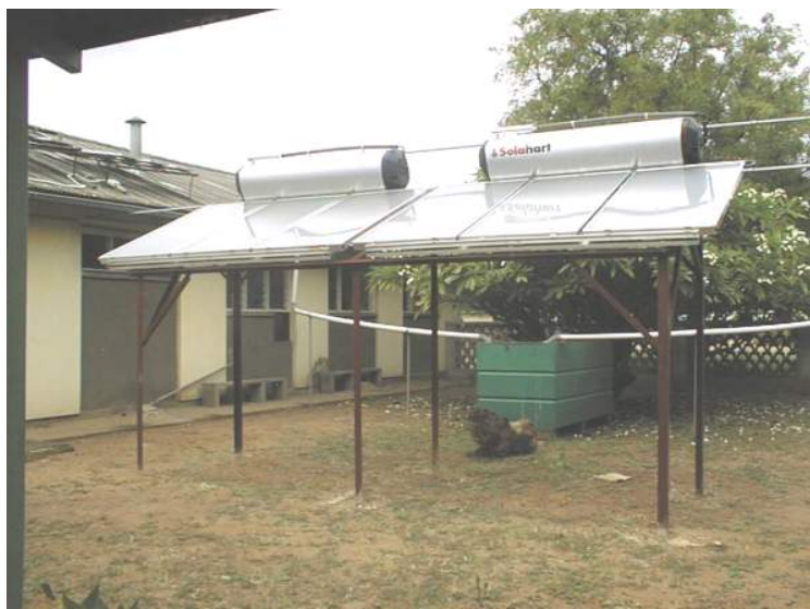
Figure 89: Indirect system with a jacket storage, Mathany Hospital, Uganda (Solahart)
