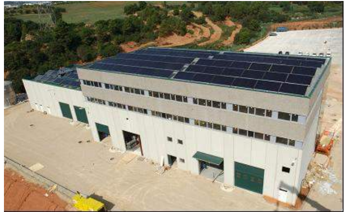
Figure 108: Parking service Castellbisbal SA, container washing, Barcelona, Spain. Installed capacity: 357 kW th . Source: Aguasol Engineering, Spain.
