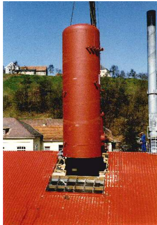
Figure 98: Installation of collectors and the 105 m 3 storage tank at the solar assisted biomass district heating plant in Eibiswald, Austria. Installed capacity 805 kW th (1150 m 2 collector area), length of district heating pipeline 4000 m.
