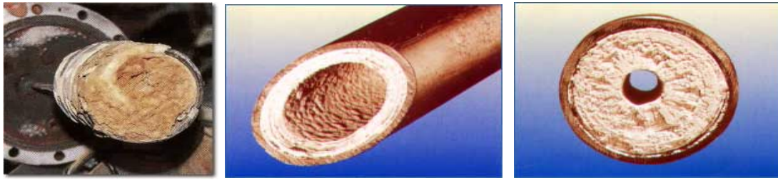
Figure 72: Calcification at a heat exchanger (left picture) and at pipes (middle and right picture) (Source: 13)
