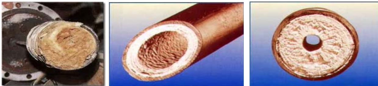
Figure 9: Calcification at a heat exchanger (left picture) and at pipes (middle and right picture) (Source: 13)
